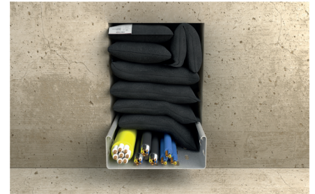
Electrical wall application
