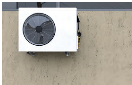
Airconditioner on the outer wall
