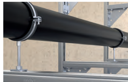
Connection on channel
