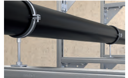
Connection on channel
