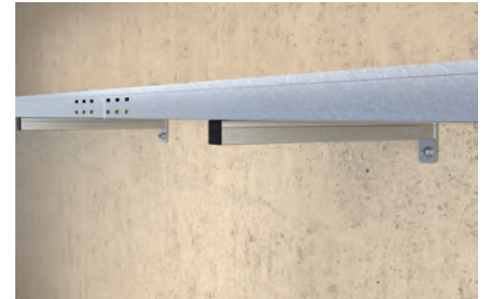
Cable tray on cantilever arm
