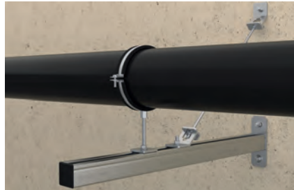
Heavy pipe on cantilever
