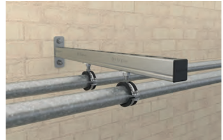
Pipelines on cantilevers
