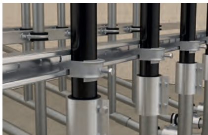
Supply lines fixed to FUS channel
