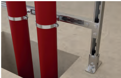
Waste water pipe
