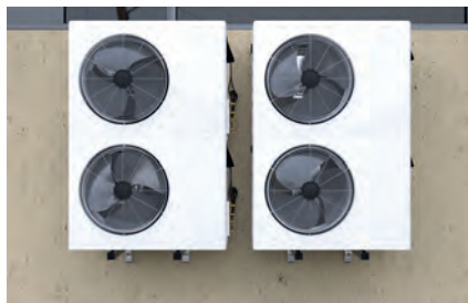
Air conditioning units
