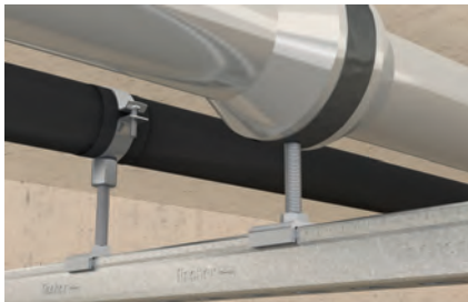
Refrigerant pipe clamps
