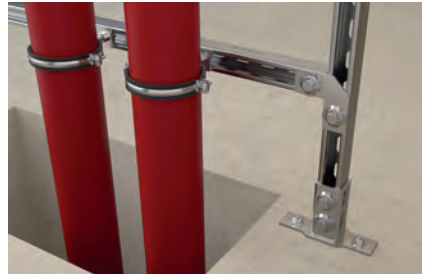
Waste water pipe
